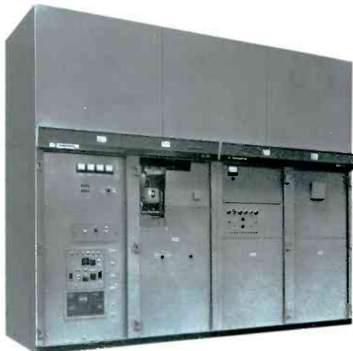
SW-50 with heat exchanger, front doors removed.
