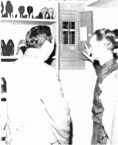
ELECTRICAL CENTER: Frank Trevarrow (right) displays load center to LBE's Joe Synar. The home is wired for 175-amp service, has 24 light circuits.
