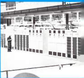
NEW SWITCHGEAR BUSINESS
