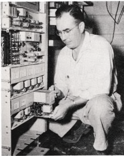
FIG. 2. Type 45A carrier system channel unit is shown being placed into position.
