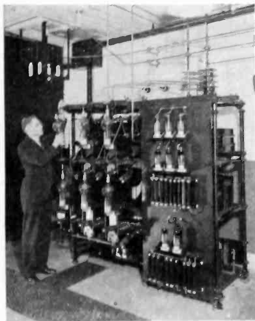
Two rectifier panels. The left hand section provides 12,000 volts at 17 amperes
