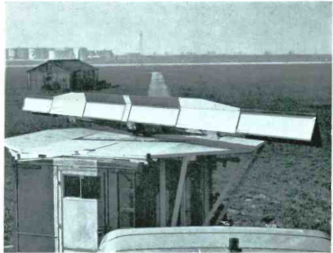
Control/Interrogator aerial installed at London Airport (Crown copyright. By courtesy of Ministry of Aviation).
