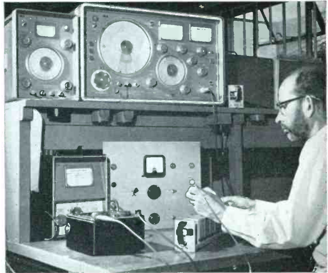
Setting up I.L.S. equipment in the Marconi test room at London Airport. The crystal oscillator output of the TF 801D/5M1 modulated to 90% by the R-C Oscillator type TF 1101 provides a test signal for a 75 Mc/s marker receiver
