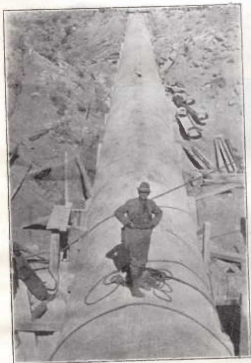
ONE OF THE STEEL PEN-STOCKS LEADING DOWN TO THE TURBINES
