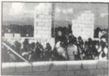
The walls are going up on the new Haiti dining room that will feed thousands of precious street children.
