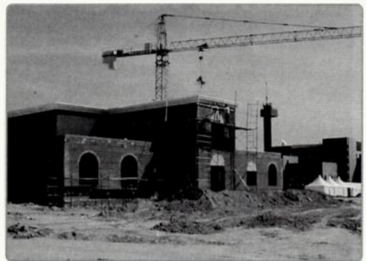
A precious TBN Partner, who is in Heaven now, is helping HER TBN build MORE STATIONS (like this studio for MADRID, SPAIN nearing completion).
