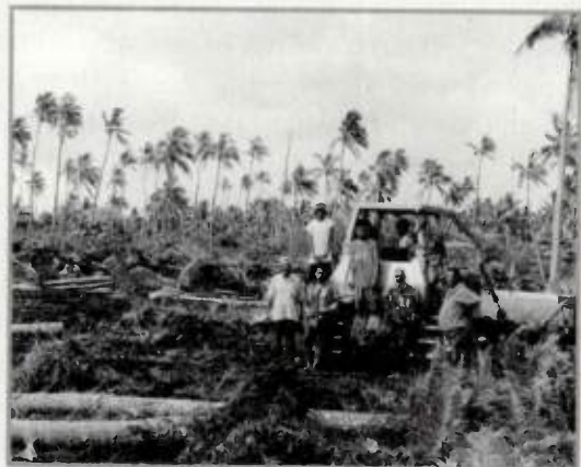
A TV station for TONGA, located in the South Pacific, is now under construction. Many precious Tongan people are volunteers, helping to build "their station." This picture was taken as they began to prepare the site where the new station will be built.
