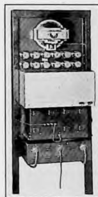
Fig. 5. Rear view of the rack installation of Fig. 4.
