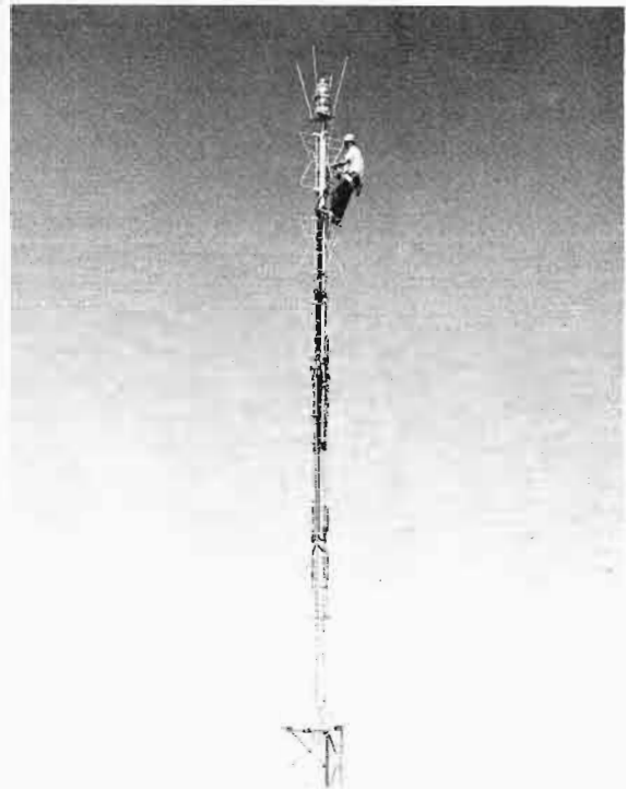
Fig. 41. Six Bay Channel 9 Superturnstile Antenna (JAMPRO Photograph).
