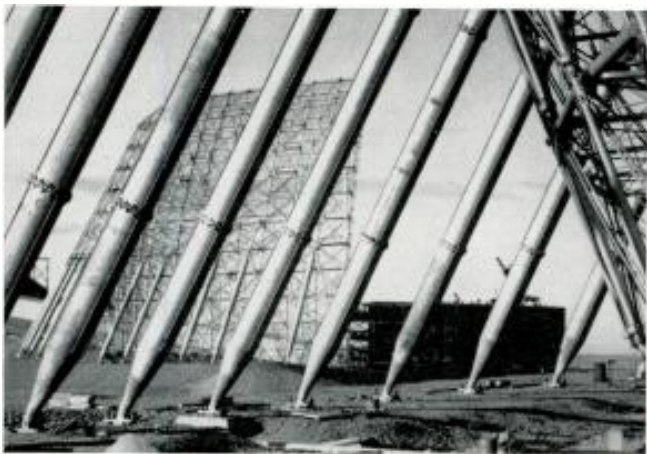
These giant antennas will withstand winds of 185 m.p.h.
