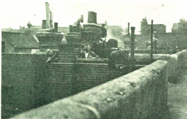
Method of wiring main group or subscribers cables in inconspicuous position. Clipped to brickwork by plugs and screws.
