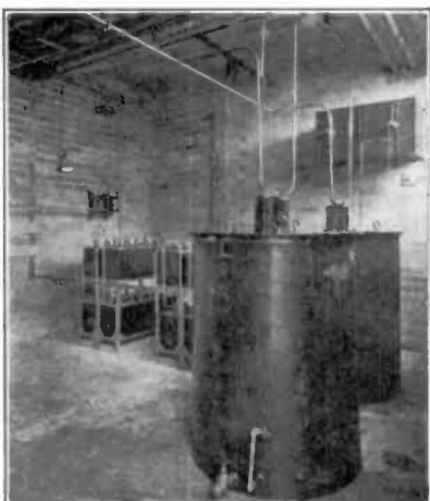
High Voltage Filter System
