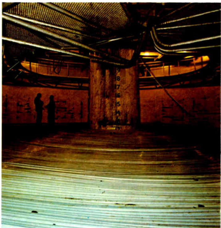
Top: arrangement of the equipment above a cable laying ship. The cable is paid out over the overhanging bow and stern sheaves at speeds of from 3 to 8 knots. Above: the No.1 cable tank aboard CS Mercury with a lightweight transatlantic telephone cable for TAT 2 (laid in 1958). For the main section of TAT 2 flexible repeaters were used, but between Newfoundland and Nova Scotia rigid repeaters were used. Right: a British designed rigid repeater passing along groups of rollers to the stern chute of CS Mercury.
