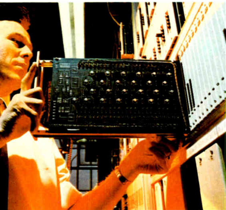
Far left: a typical multi-pair cable may contain up to 4800 pairs. This is laid underground. It is terminated on a distribution frame in the exchange and split into smaller cables en route which terminate at distribution points. From here single pairs connect private telephones. Left: testing uniselectors in Strowger exchange equipment. Above: a reed relay/electronic exchange. Electronic techniques are used to control the reed relay function. Such systems are reliable, fast, and flexible.
