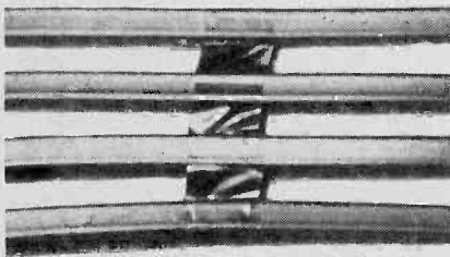
Short lengths of electrical tape help space out the twin-leads to keep them isolated and to support them in place properly.
