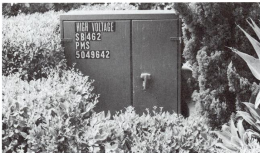
Fig. 9 Ground-mounted transformer can be a serious source of RFI.
