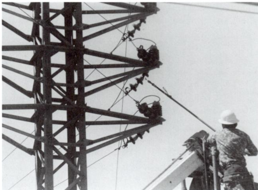
Fig. 3 The source of RFI has been spotted by the investigator and he has summoned a lineman to place a RIV clip in between a string of bell insulators. Basic knowledge of power line construction and radio communication is an important combination required by the RFI investigator. Individuals with a basic education in electronics can be trained in this new and expanding field.
