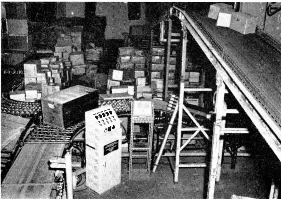
This shows the control equipment console and the five photoelectric heads for the conveyor system of Fig. 1
