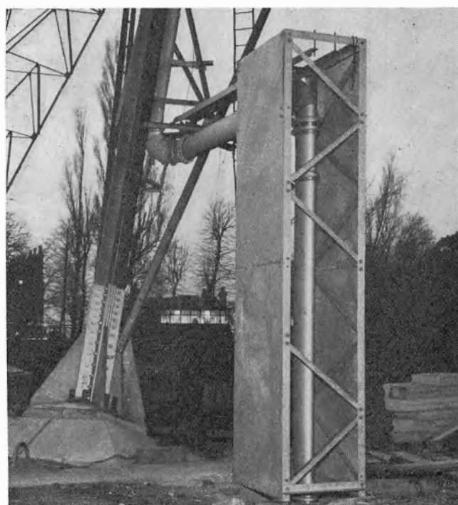
Fig. 2. The elliptical waveguide at the front of the tower showing the concertina expansion couplings and the construction of the angle bends. The partly constructed cover is designed to protect the waveguide from mechanical damage
